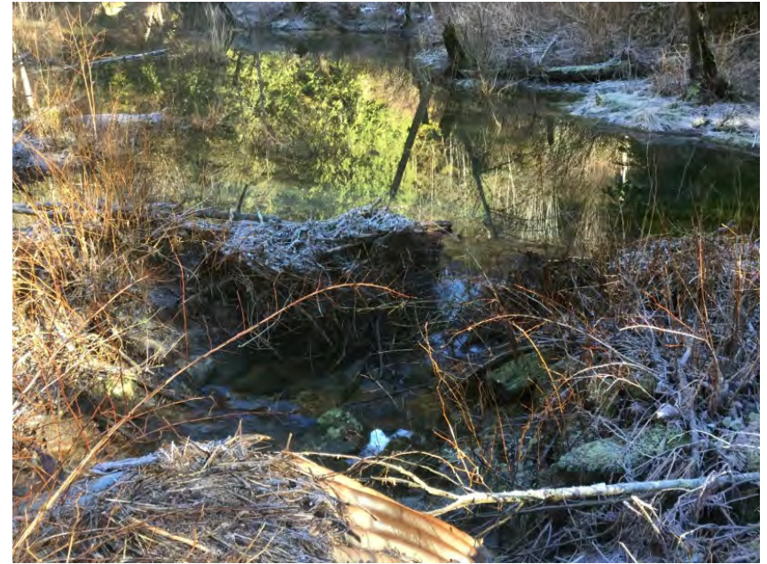
Inlet debris, see material on top of the culvert
